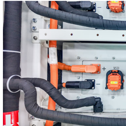
prefabricated energy storage cabin and power grid
