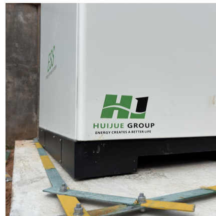
Deploying Battery Energy Storage Solutions in Tunisia
