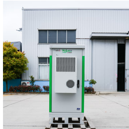
Containerized energy storage , Microgreen.ca
