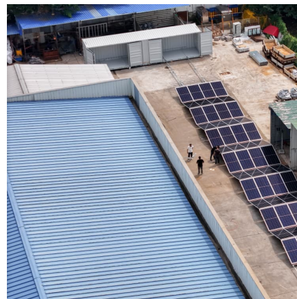
Energy storage container. BESS container
