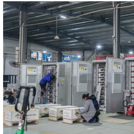
Commercial Battery Storage , Electricity , 2023 , ATB
