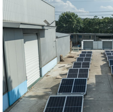
Utility-Scale PV , Electricity , 2024 , ATB , NREL
