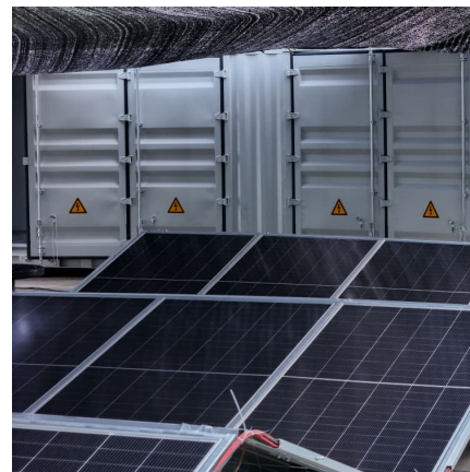
Hybrid power plants, solar+storage were big in 2022, ...
