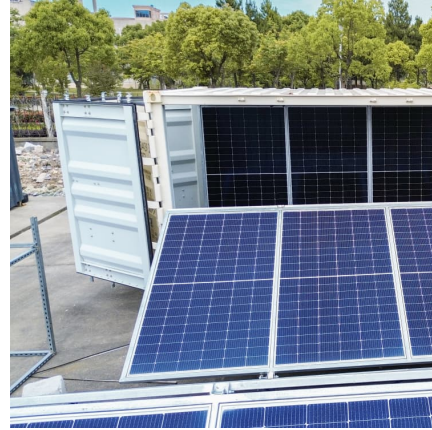
Containerized energy storage . Microgreen.ca
