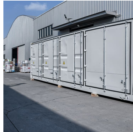
Energy storage container, BESS container
