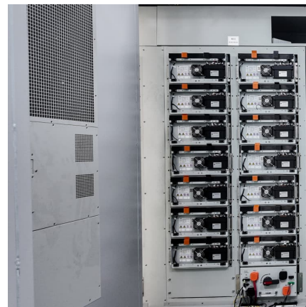
Ouagadougou energy storage plant operation
