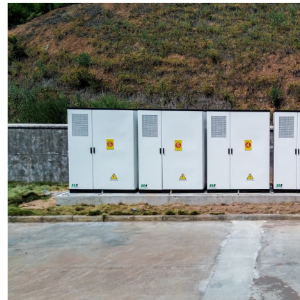
Battery energy storage system (BESS) container. ...
