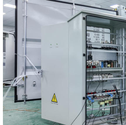
Containerized Maritime Energy Storage , ABB Marine ...
