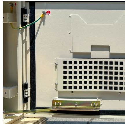
Malabo fengqiao energy storage power station
