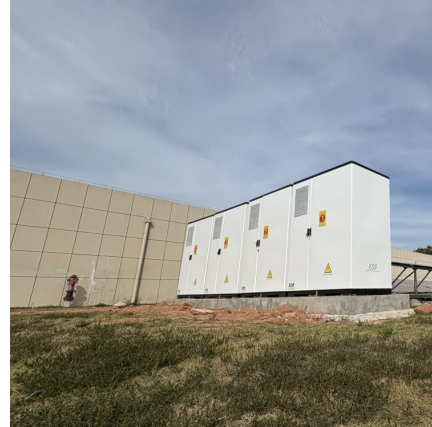
Malabo fengqiao energy storage power station
