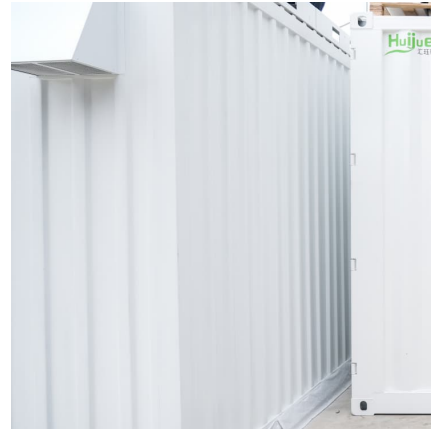
Luxembourg city air energy storage power station
