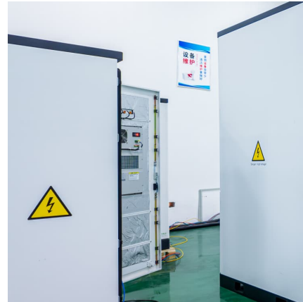
Photos of modern energy storage charging piles
