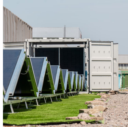
oceania photovoltaic energy storage plant
