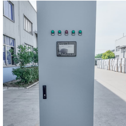
ouagadougou container energy storage power station
