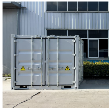
Container energy storage device in ouagadougou
