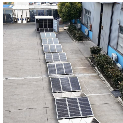
Sao Tome Photovoltaic Energy Storage Power Station
