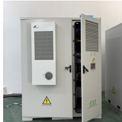
Commercial energy storage device in ouagadougou
