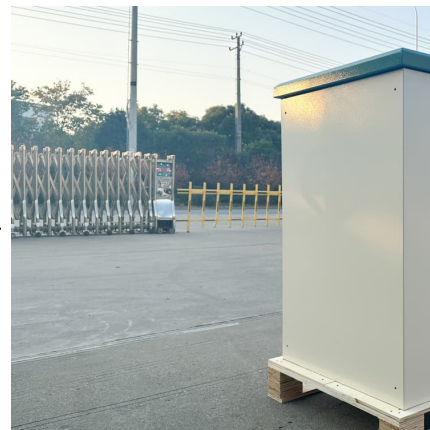
Croatia commercial energy storage system
