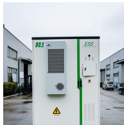
Wall-mounted Battery ?BSLBATT
