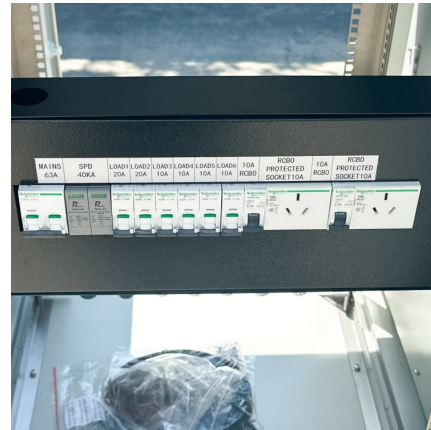
port of spain containerized energy storage system
